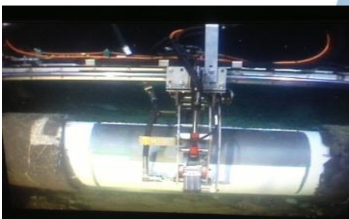
Coating Removal System
